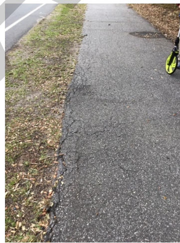
Figure B – Edge Cracking
