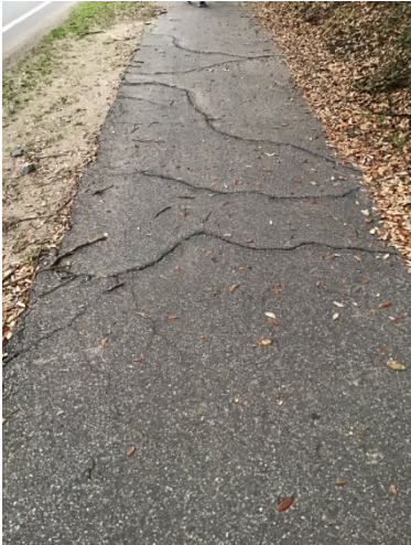
Figure C – Root intrusion cracks
