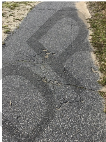
Figure A - Transverse Cracking
