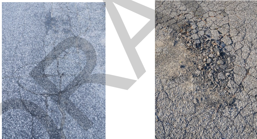
Figures 3 & 4: Fatigue Cracking as seen on First Avenue and Mizzen Mast
