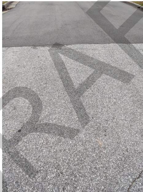
Figure 9: Oxidation versus newer pavement (top of picture)
