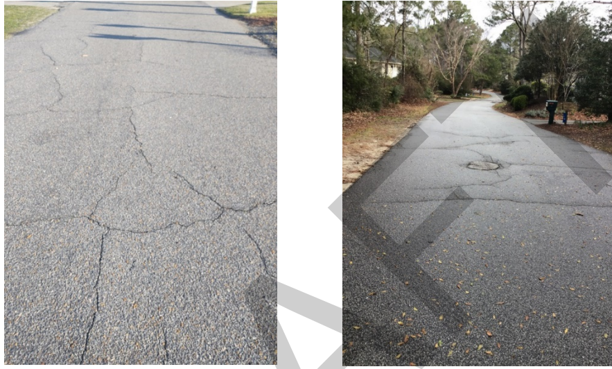
Figures 5 & 6: Block Cracking and Transverse Cracking as seen on Ocean Boulevard and Ginguite Trail
