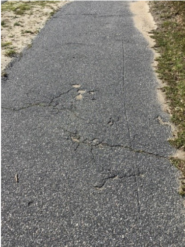
Figure A - Transverse Cracking
