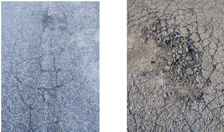
Figures 3 & 4: Fatigue Cracking as seen on First Avenue and Mizzen Mast
