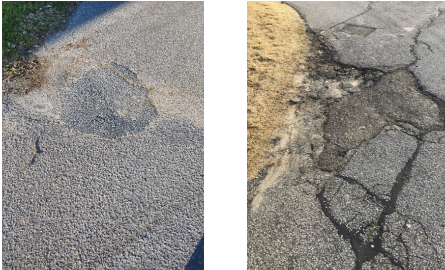
Figures 7 & 8: Patching that is failing (patches sinking and cracking)
