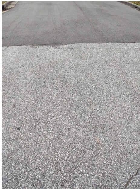
Figure 9: Oxidation versus newer pavement (top of picture)
