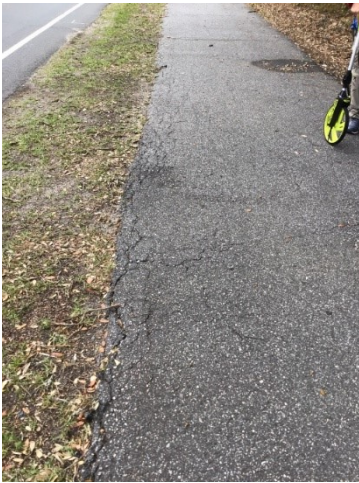
Figure B – Edge Cracking
